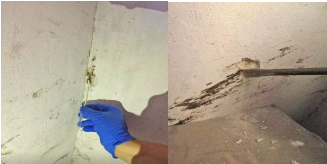
FIGURE 4: SAMPLING OF SPLATTER OF BLACK SUBSTANCE ON INDOOR WALLS IN MAREA
