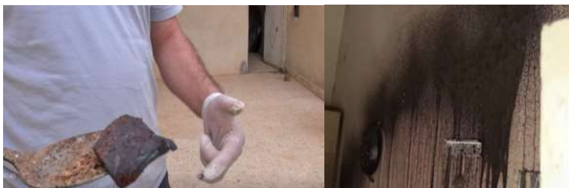
FIGURE 5: SAMPLING OF SOIL CONTAMINATED BY BLACK, OILY SUBSTANCE IN AN IMPACTED BUILDING IN MAREA ON 9 SEPTEMBER 2015 (LEFT); SPLATTER OF THE BLACK LIQUID ON THE WALL OF THE IMPACTED BUILDING (RIGHT)
