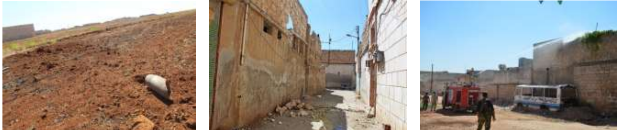
FIGURE 16: IMPACT DAMAGE, TYPICAL OF INERT ARTILLERY PROJECTILES, AS OBSERVED AT THREE LOCATIONS
